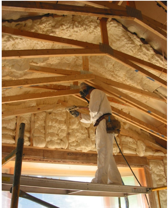
Brad Eisele, manager of Arbor Insulation, sprays soybean-based insulation in a home near Dexter.
